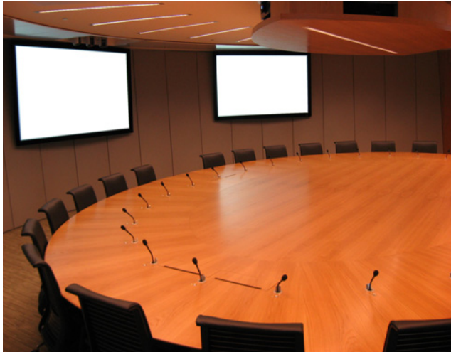
Corporate board room in Australia using AV-M8s to move audio from the conference mics to an equipment room
