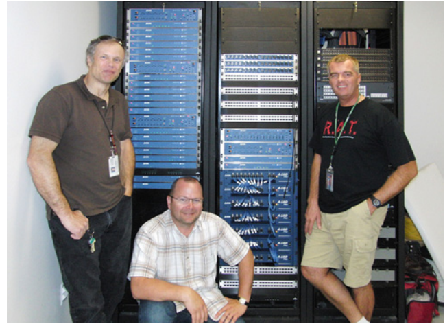
Tommy Wiggins, Aviom's Jeff Lange, and Mark Baker in the Tri-C machine room with the Aviom sub-networks and SMPTE network
