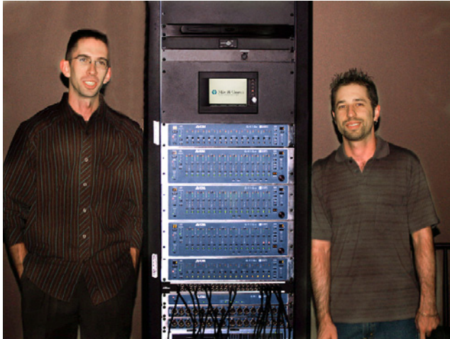
Andrew Welker, field engineer installer for Ford Audio-Video, and Nathan Marschall, head audio engineer at Mile Hi Church
